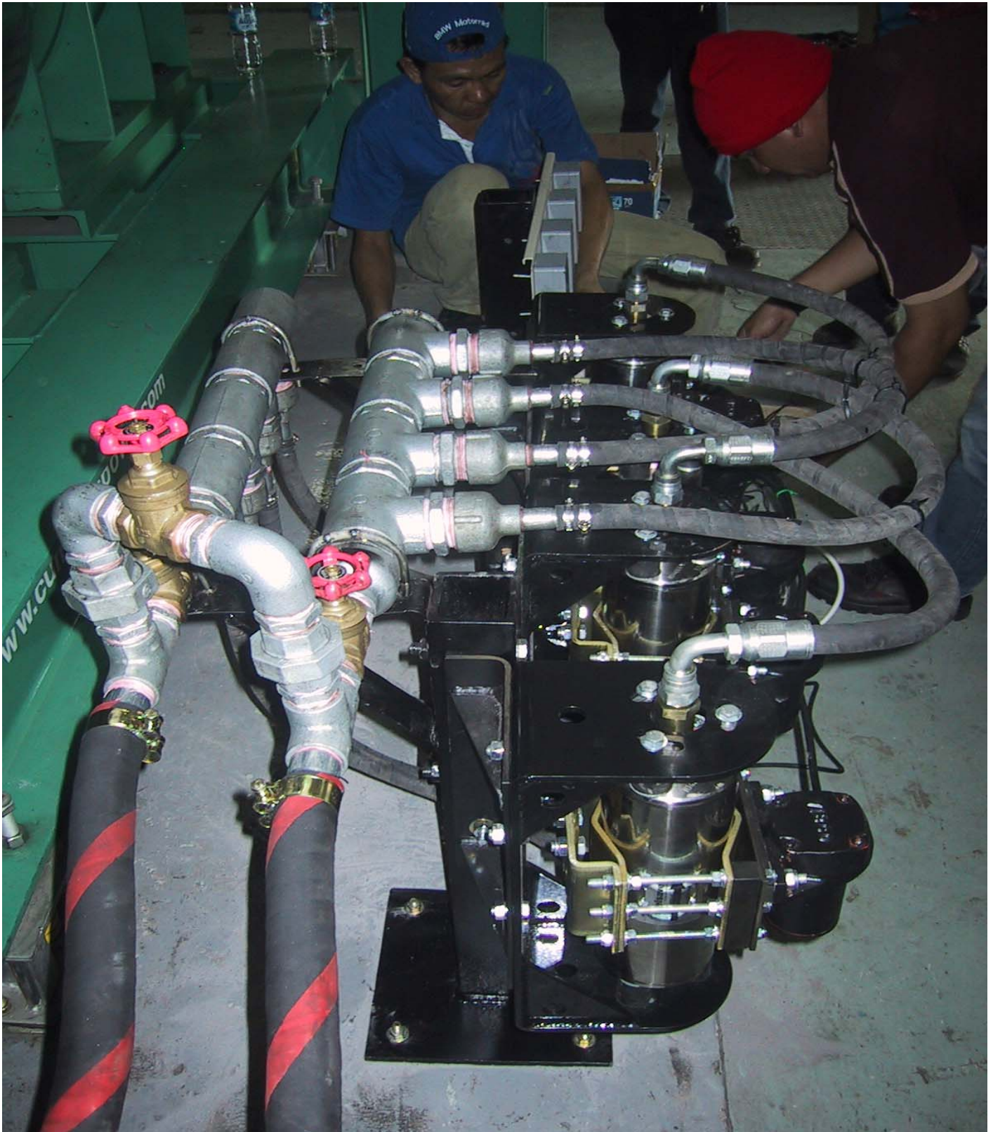
Pic 2.... 4 x ID400EV Fuelstars with manifolding & bypass
