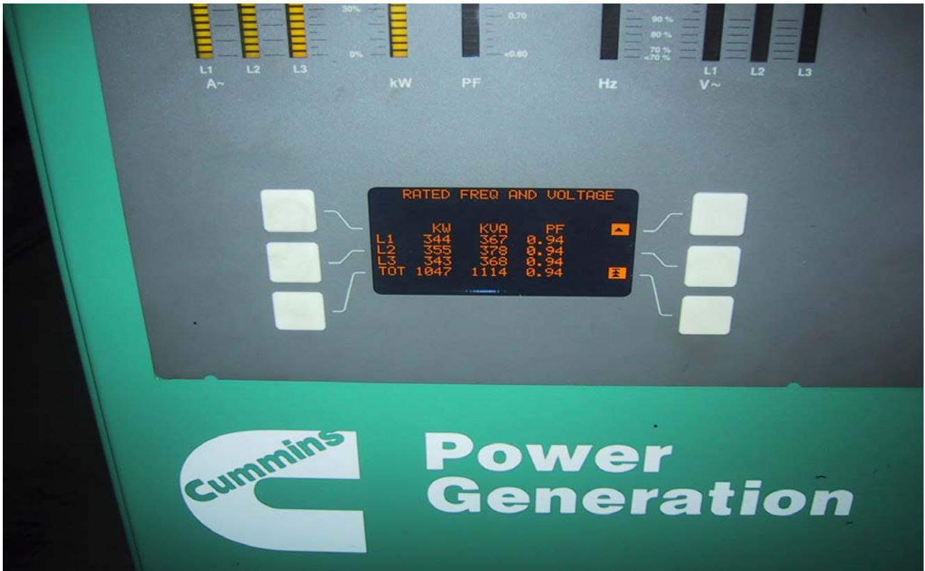
Pic 3 .....Control panel before Fuelstar installation
